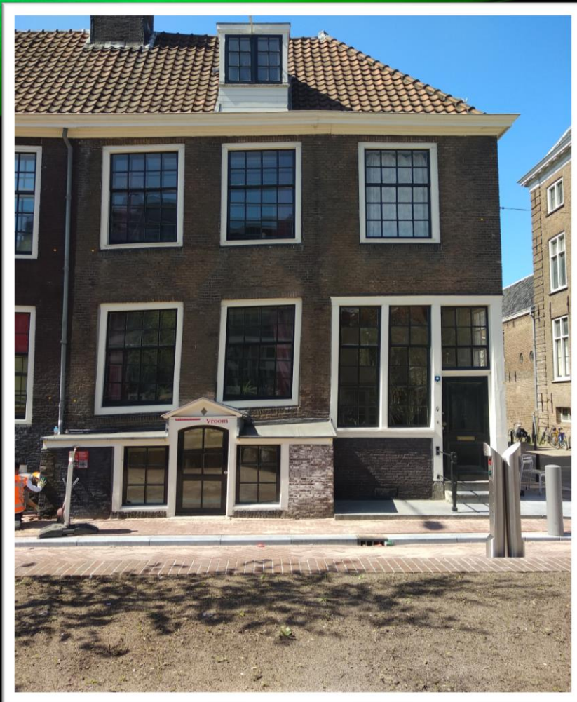
Heritage house Impacted by settlement due to leakage
